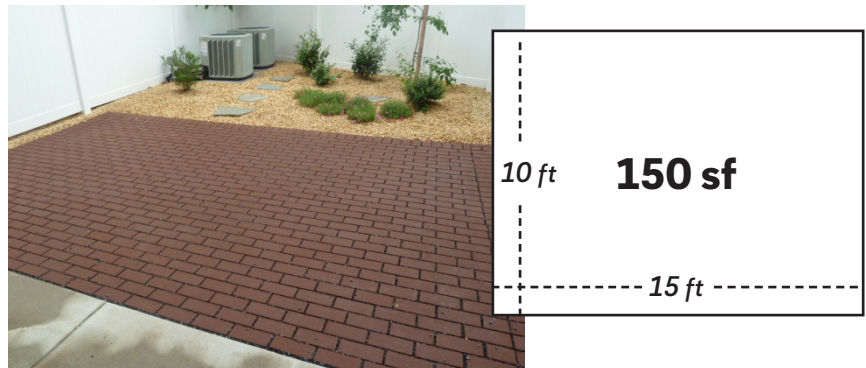
This patio had 150 sf of concrete removed and replaced with permeable pavers. Access to the space was easy.
